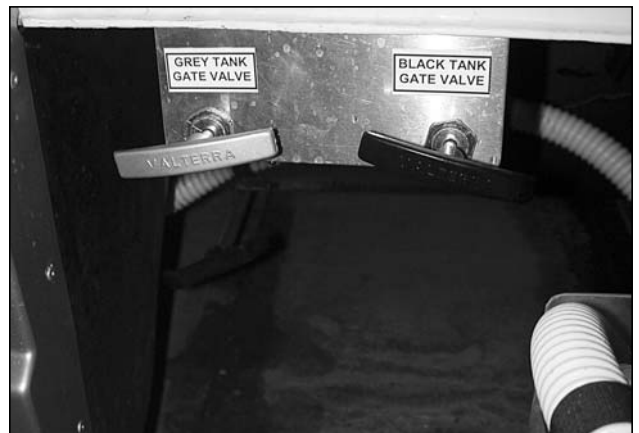
Picture G-P14: Access to sewer discharge assembly, black and grey gate valve handles.
