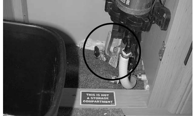
Picture G-P6: Interior tank drain valve in open position.
