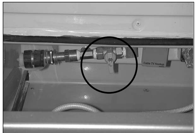
Picture G-P12: Closed position of the city water tank fill valve.
