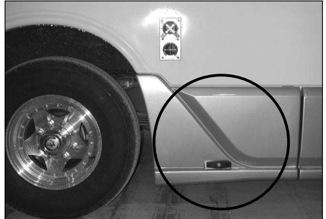
Picture B-P34: Auxiliary battery compartment.
