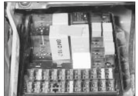
3.3b Fusebox cover removed to expose fuses and relays (1.8 CVH model shown)
