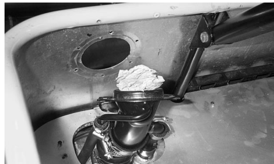
Figure 189: Old filler boss removed
