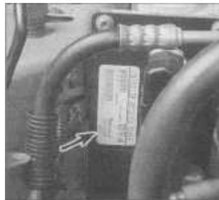
2.2 The Controller Anti-lock Brake (arrow) is the brain of the ABS system (1997 and earlier style shown; on 1998 models, the CAB is mounted on the HCU)
