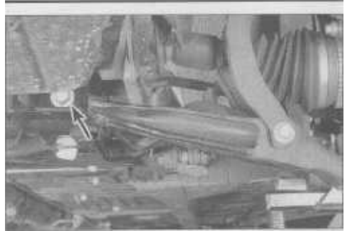
6.12b . . . and the pivot bolt holding the front of the lower control arm to the front suspension crossmember
