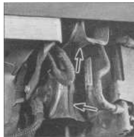
21.12 The horns (arrows) are located behind the front bumper on the right side frame rail, one above the other
