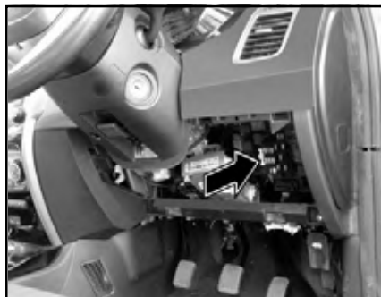
Fuse Box - Cabin Compartment
