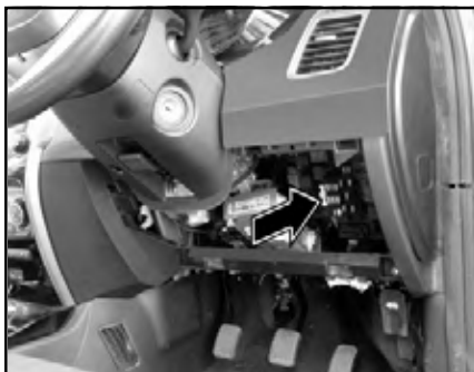
Fuse Box - Cabin Compartment
