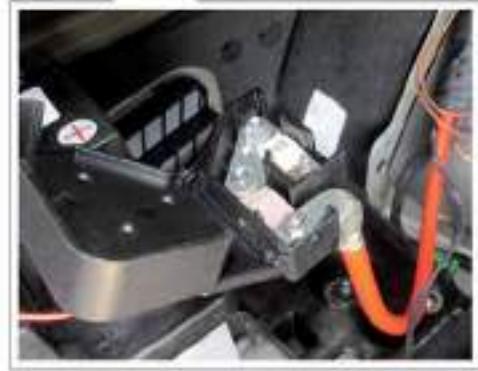
Fuse (200 A) on positive terminal of 12-volt vehicle battery
