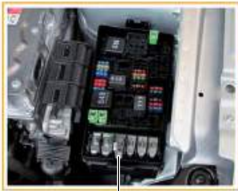
Electronics box with relay and fuse holder SB and multifuse pre-fuse holder SA
